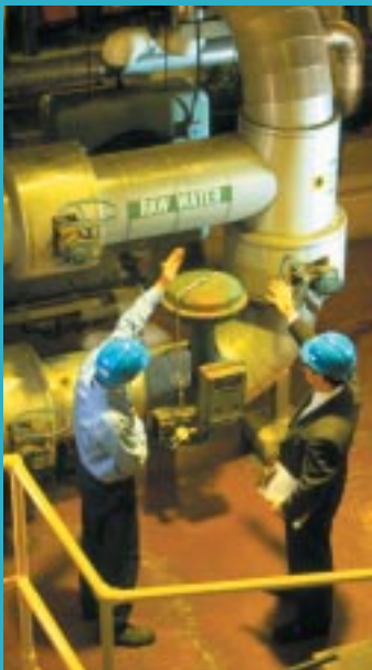
Patrick Williams, maintenance manager, and Stuart Nachmias, project manager, discuss water flow characteristics at Waterside Steam Station.
