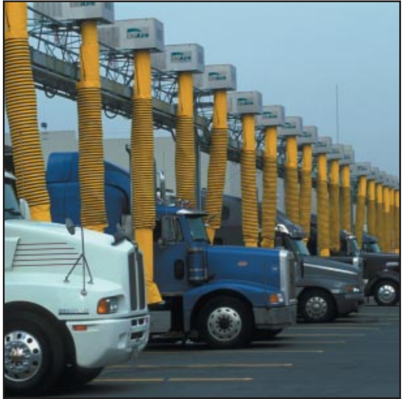
At the truck stop electrification project at Hunts Point Cooperative Market, drivers can enjoy air conditioning in their cabs and maintain refrigeration without idling their motors.
