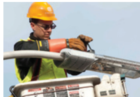
LED streetlight being installed in Cresskill, New Jersey, by Orange and Rockland line technician.
